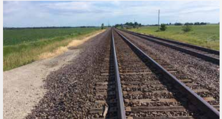
Tracks treated using the Cleantraxx™, Opensight® and Spike 80DF® herbicides bareground mix in southern Illinois.
